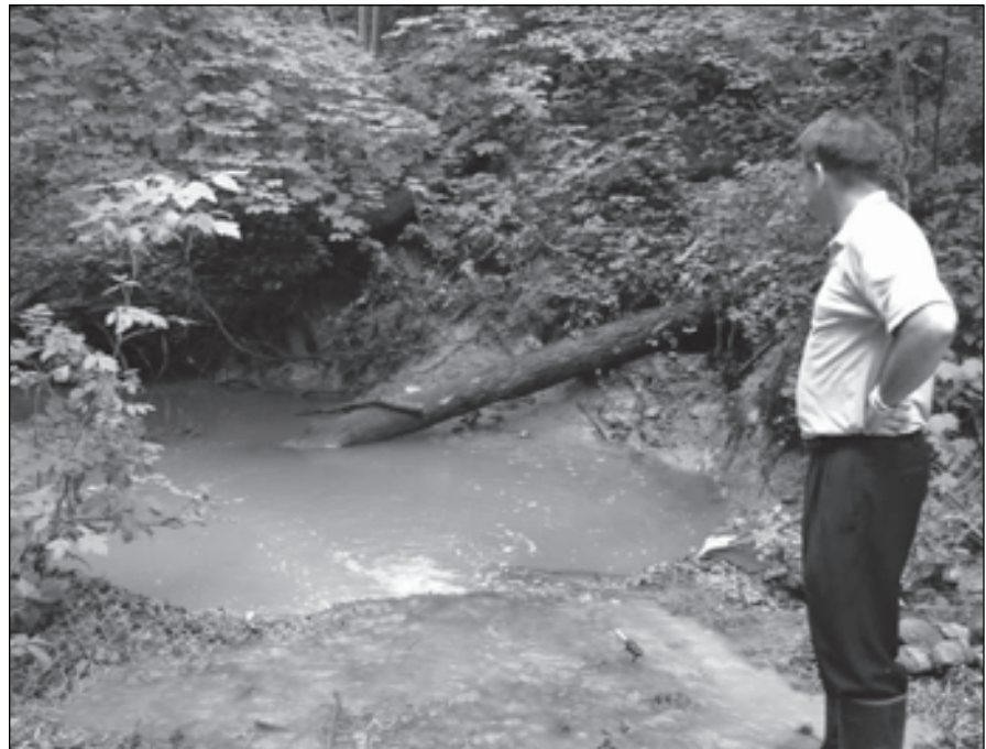
Figure 15. Reno mattress streambed armor installed over a layer of filter cloth in eroding bed of Ravine 10. Note streambed erosion scour and flanking on right (2007 photo).
