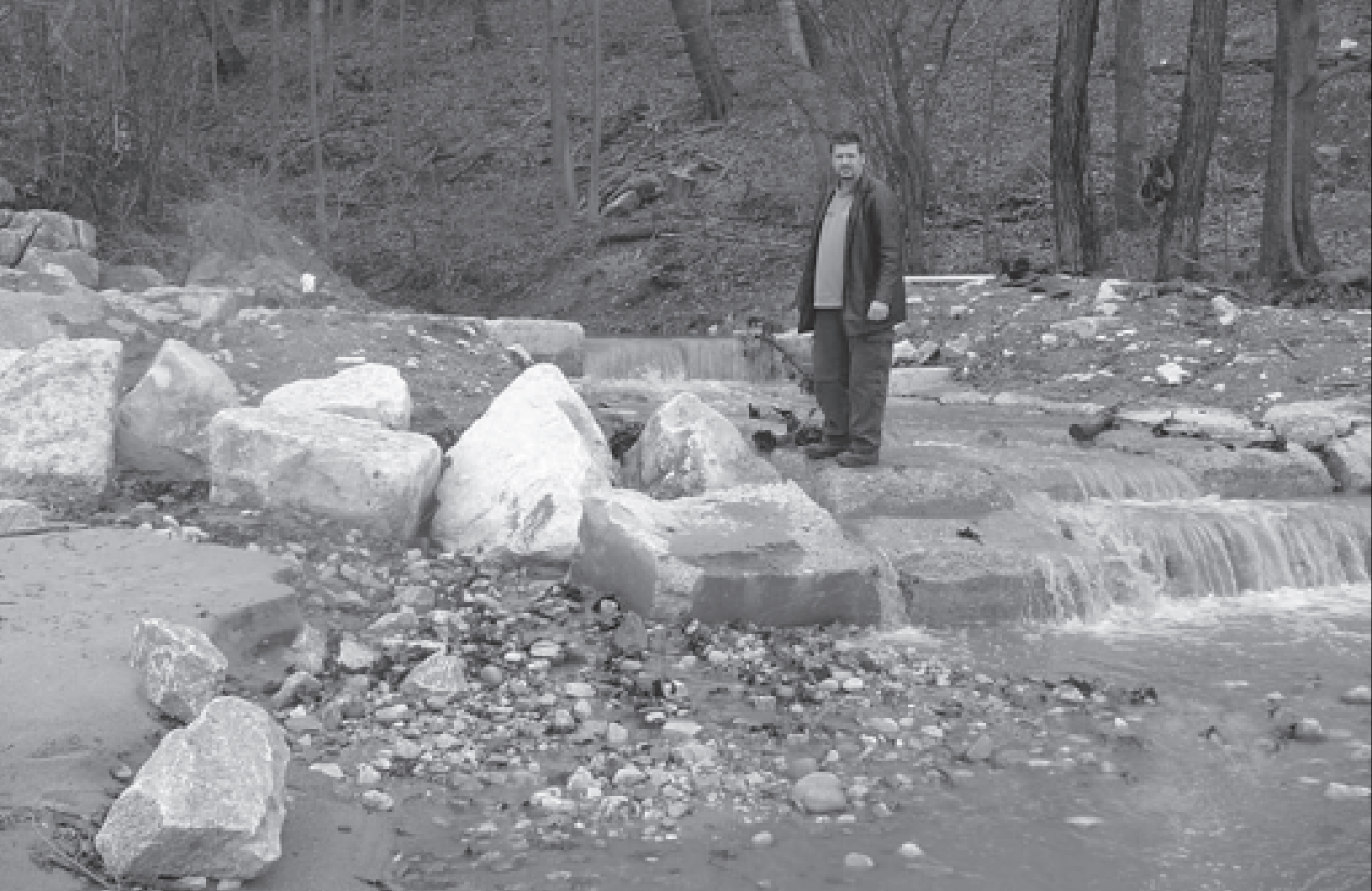
Figure 22. Glencoe Ravine. Newly constructed east check dam after rainstorm (3 May 2004 photo). Falls have added benefit of aerating the stream water.
