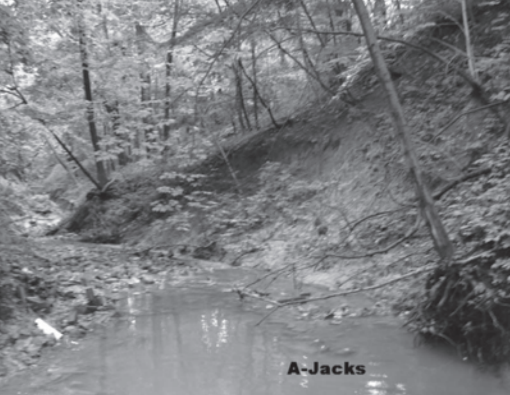
Figure 17 (top). A-Jacks streambank armor flanked after 15 years. Structural integrity of system is lost because of high stream flow velocities and scour. Note eroded slope has retreated approximately 2.5 feet back from row of A-Jacks (2007 photo).
