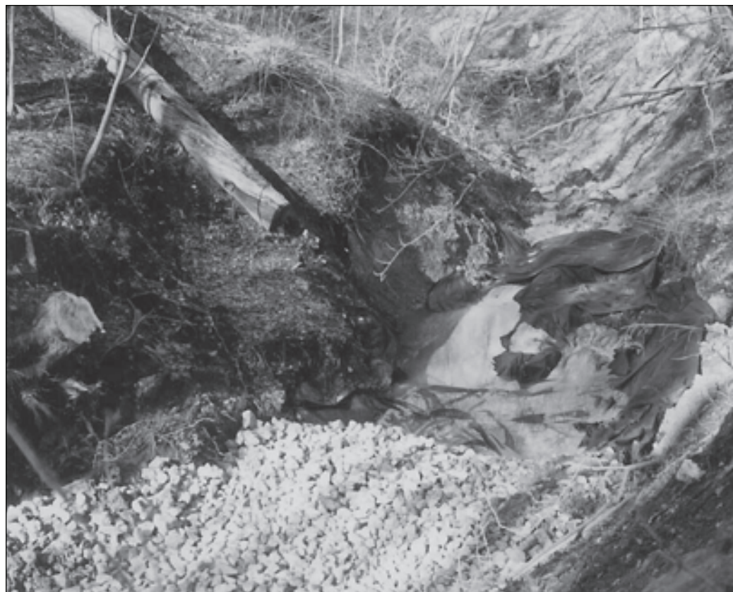
Figure 4. Ravine Park Ravine streambed and banks repaired with a 3-foot-thick layer of 6-inch to 12-inch limestone (stream armor) over geotextile (1992 photo). Concurrently, slumps were filled with limestone and concrete rubble and covered with hydroseeded soil. A subsequent survey showed that it took approximately one year for the void space between the new stream cobbles to fill with sand and gravel eroded from upstream slumps.
