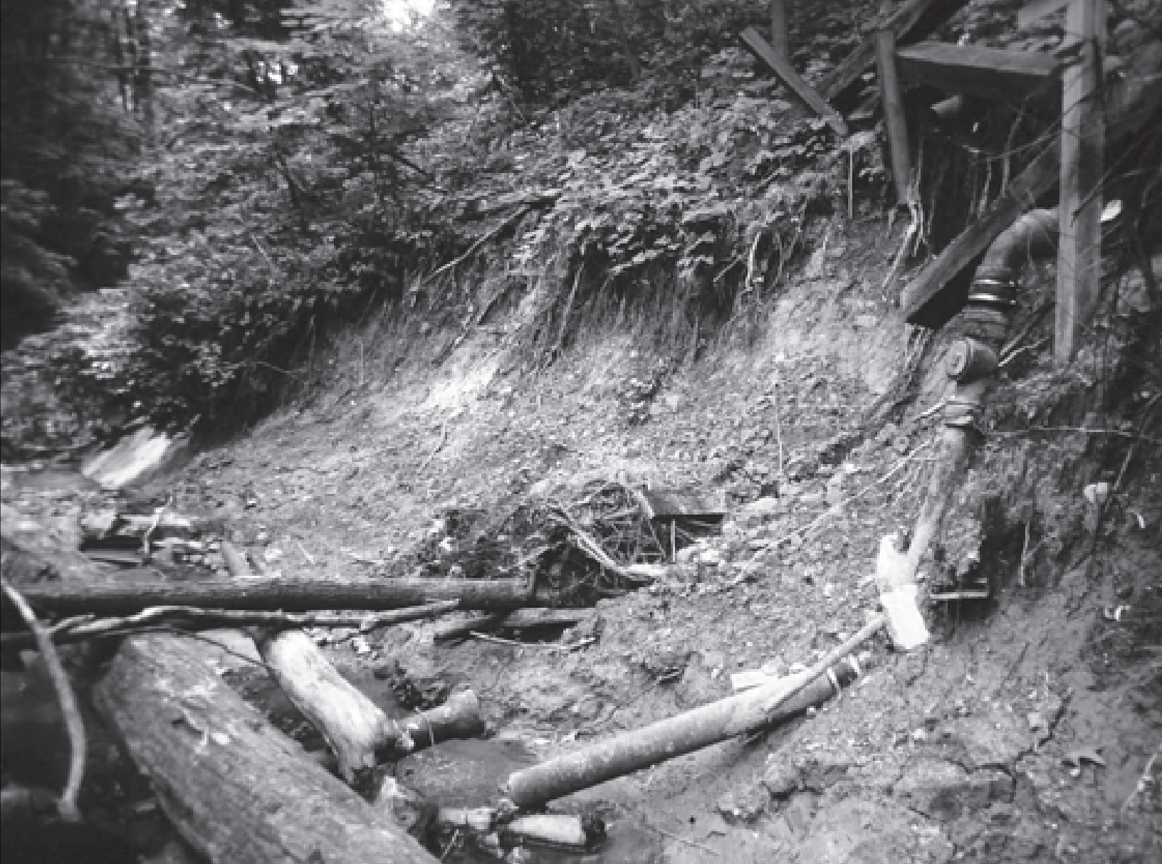
Figure 10. Ravine 10, city of Highland Park, Illinois. Unrestored ravine with active streambed erosion and slope failure. Broken sanitary sewer can be seen at the lower center (1992 photo).
