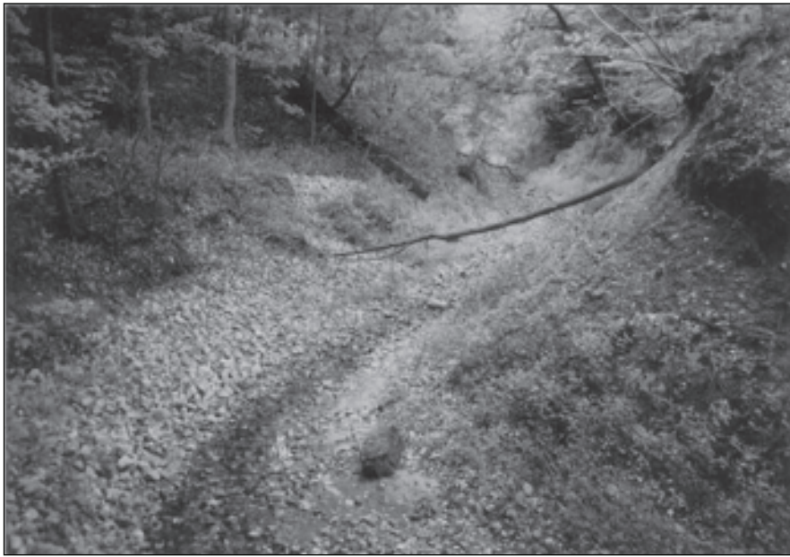
Figure 5. Ravine Park Ravine four years after construction. Stream flow is now visible on the surface. In prior years, the water flowed below the top of the stone work. Note encroachment of vegetation over the new stone and steep slope on right that has not fully vegetated.
