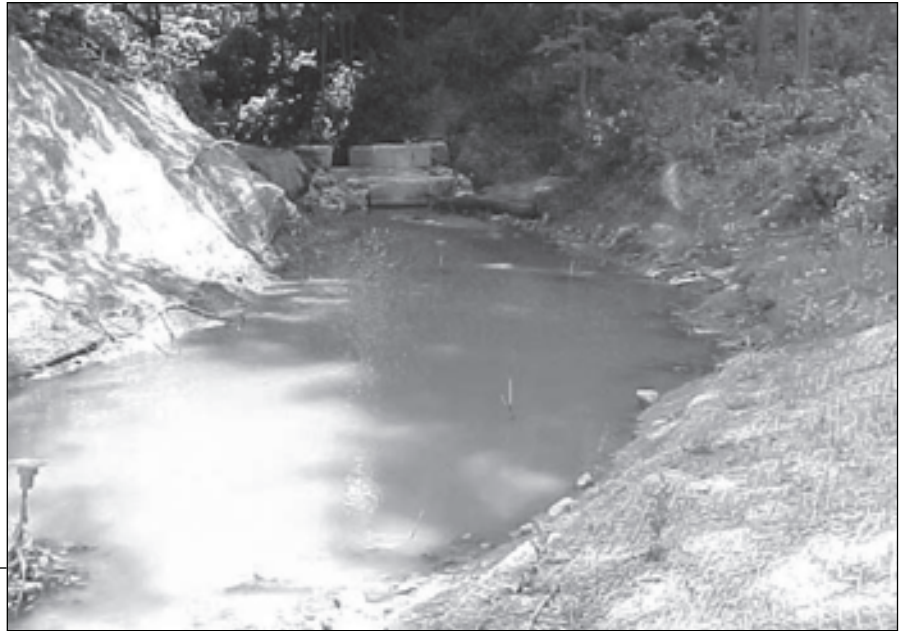
Figure 23 (top). New east retention pond in Glencoe Ravine with erosion cloth and new plantings (upper check dam in background). Note steel survey rods (20 October 2004 photo).
